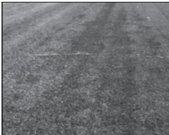
Figure A-12h. Porous Friction Course Medium-Severity Raveling and Weathering
