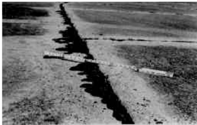
Figure B-11b. Medium-Severity Settlement on Apron
