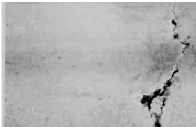
Figure B-3c. High-Severity Crack
