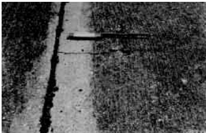
Figure B-13a. Shrinkage Crack
