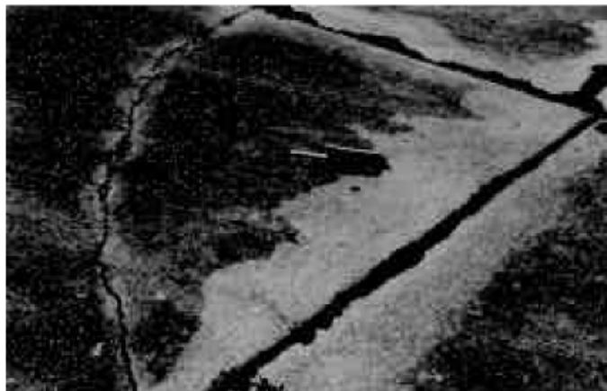
Figure B-2b. Medium-Severity Corner Break
