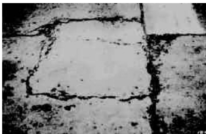
Figure B-7c. High-Severity Patching, Large
