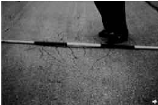
Figure A-5b. Medium-Severity Depression
