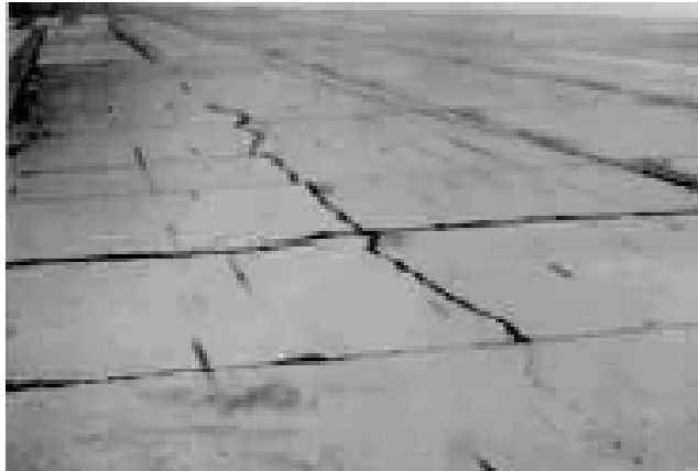
Figure B-12a. Low-Severity Intersecting Cracks
