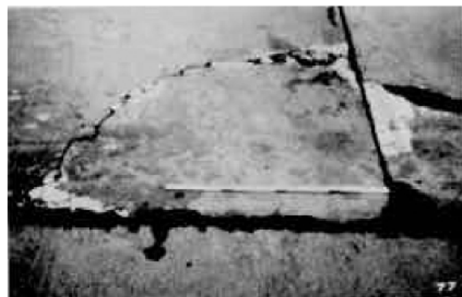
Figure B-2c. High-Severity Corner Break
