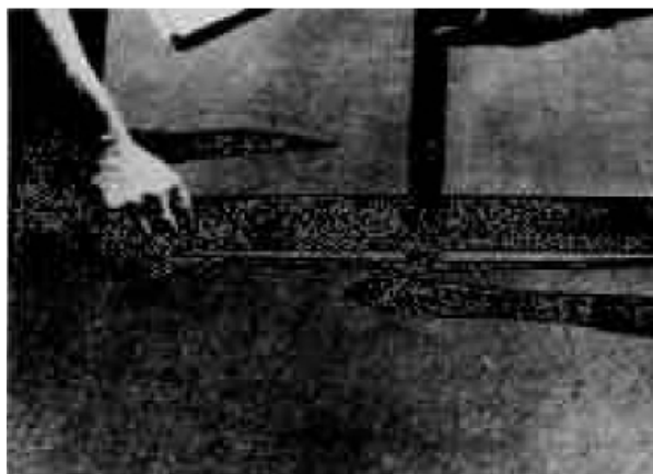
Figure A-13b. Medium-Severity Rutting
