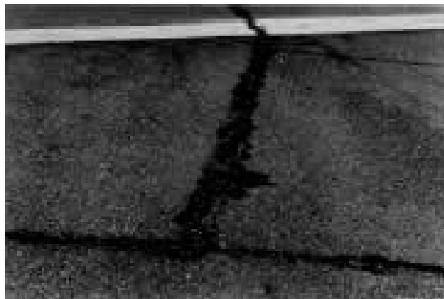
Figure A-7c. High-Severity Joint Reflection Cracking
