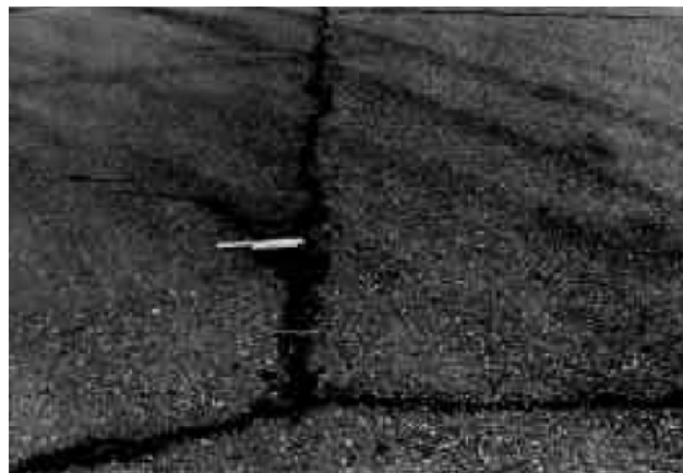
Figure A-7b. Medium-Severity Joint Reflection Cracking
