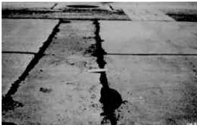
Figure B-7b. Medium-Severity Patching, Large
