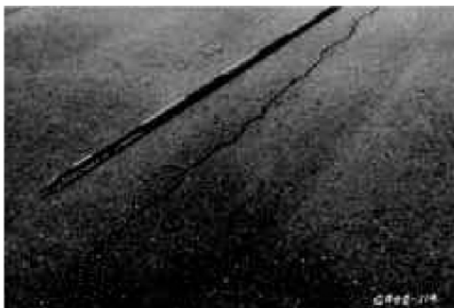
Figure A-8b. Medium-Severity Longitudinal and Transverse Cracking
