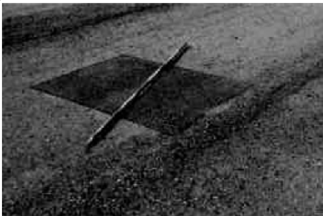
Figure A-10a. Low-Severity Patching and Utility Cut Patch
