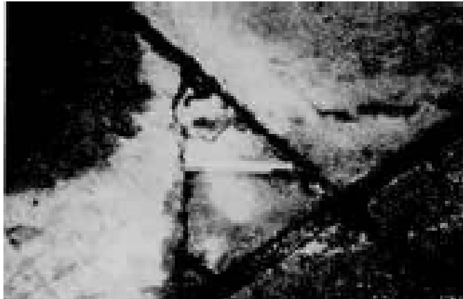
Figure B-15b. Medium-Severity Corner Spall
