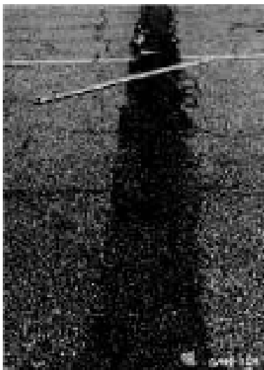
Figure A-10b. Medium-Severity Patching and Utility Cut Patch
