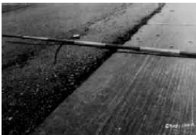
Figure A-14b. High-Severity Shoving
