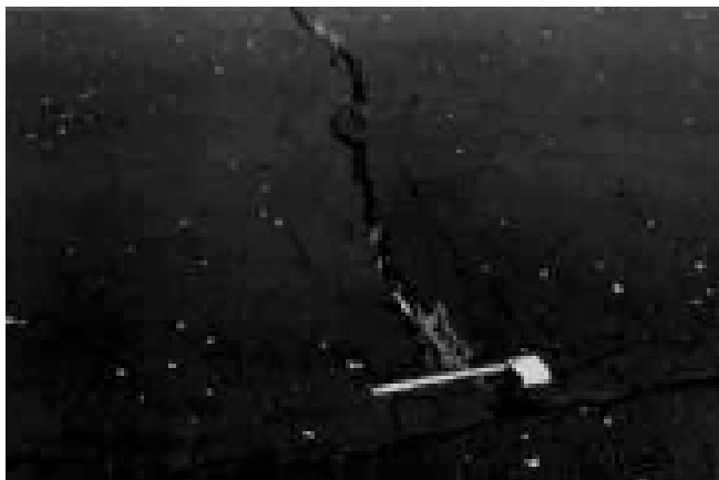
Figure A-8c. High-Severity Longitudinal and Transverse Cracking
