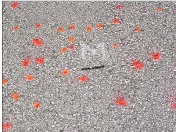
Figure A-12b. Dense Mix Medium-Severity Raveling and Weathering
