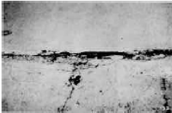
Figure B-14c. High-Severity Joint Spall
