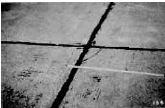
Figure B-15a. Low-Severity Corner Spall
