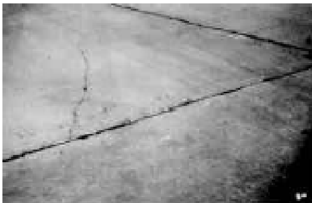
Figure B-3a. Low-Severity Diagonal Crack
