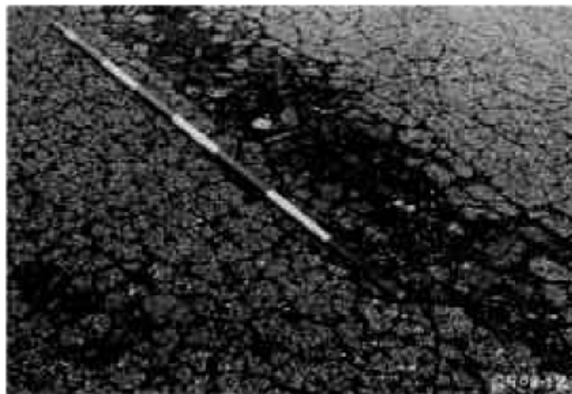
Figure A-1c. High-Severity Alligator Cracking
