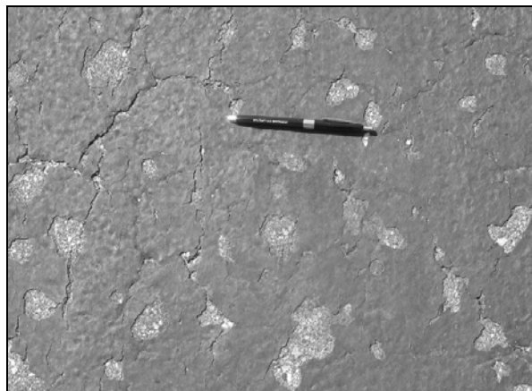
Figure A-12f. Tar over Dense Mix High-Severity Raveling and Weathering
