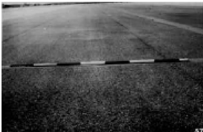
Figure A-13a. Low-Severity Rutting
