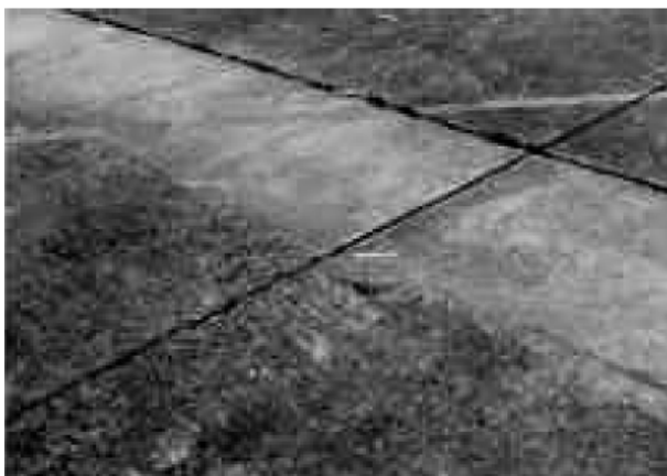
Figure B-4a. Low-Severity Durability Cracking
