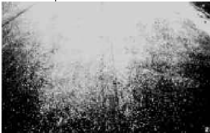
Figure A-4. Corrugation
