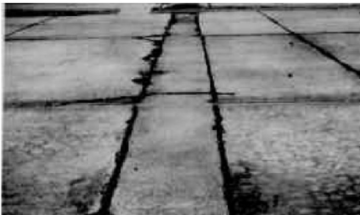
Figure B-7a. Low-Severity Patching, Large
