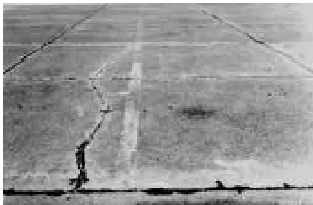
Figure B-3b. Medium-Severity Longitudinal Crack
