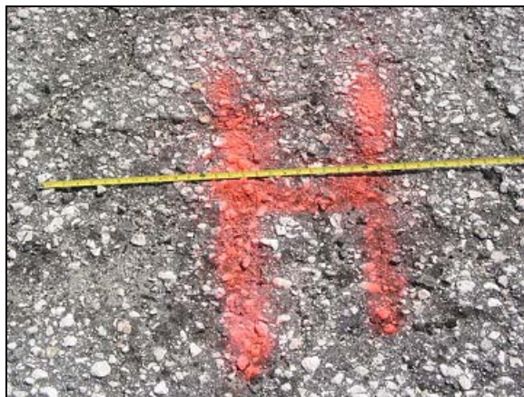
Figure A-12c. Dense Mix High-Severity Raveling and Weathering
