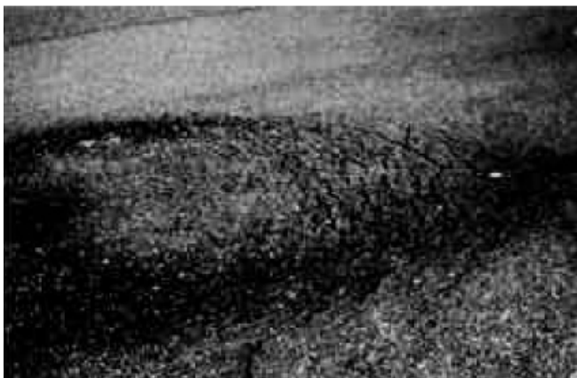
Figure A-15a. Slippage Cracking
