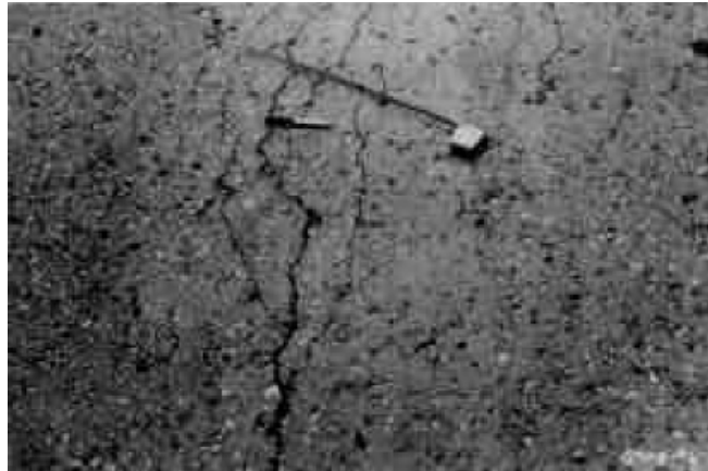
Figure A-1a. Low-Severity Alligator Cracking
