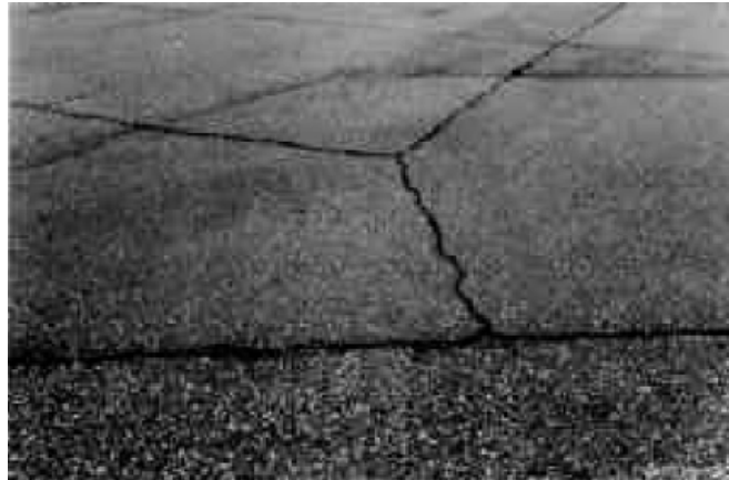
Figure A-7a. Low-Severity Joint Reflection Cracking
