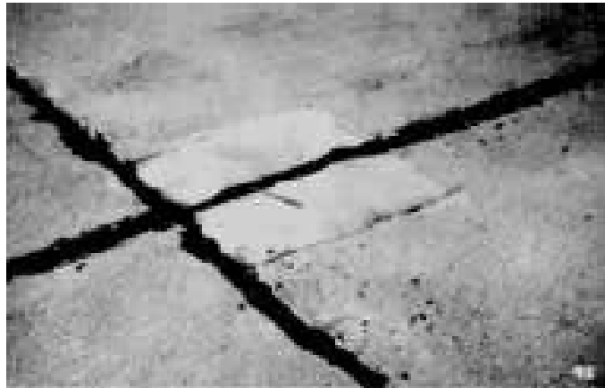
Figure B-6a. Low-Severity Patching, Small
