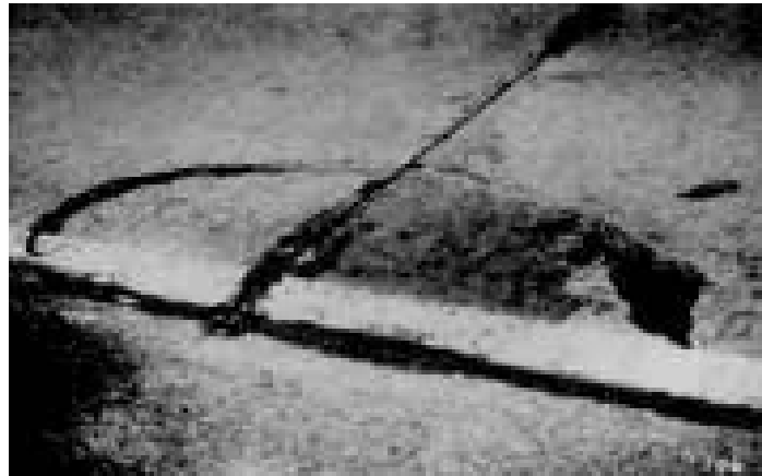
Figure B-9a. Pumping (note fine material on surface that has been pumped and has caused corner break)
