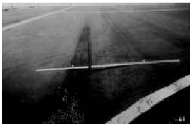
Figure A-13c. High-Severity Rutting
