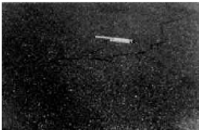
Figure A-8a. Low-Severity Longitudinal and Transverse Cracking
