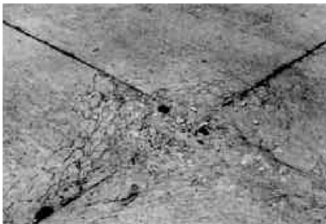
Figure B-4c. High-Severity Durability Cracking
