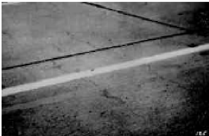
Figure B-13b. Shrinkage Cracks
