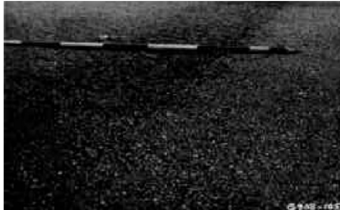
Figure A-5a. Low-Severity Depression
