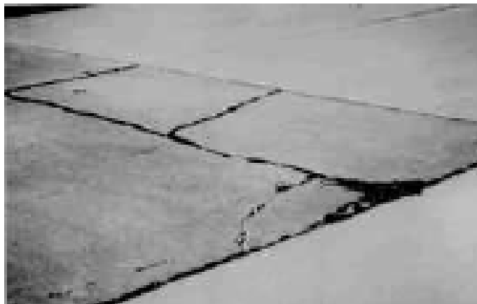
Figure B-12b. Medium-Severity Intersecting Cracks
