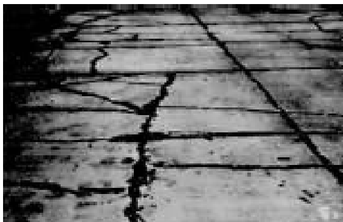
Figure B-12c. Shattered Slab
