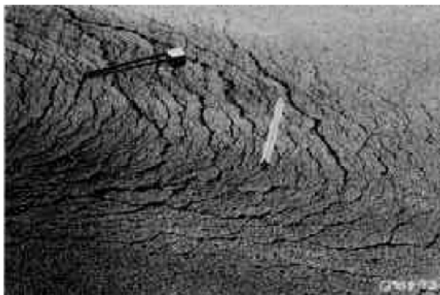
Figure A-15b. Slippage Cracking
