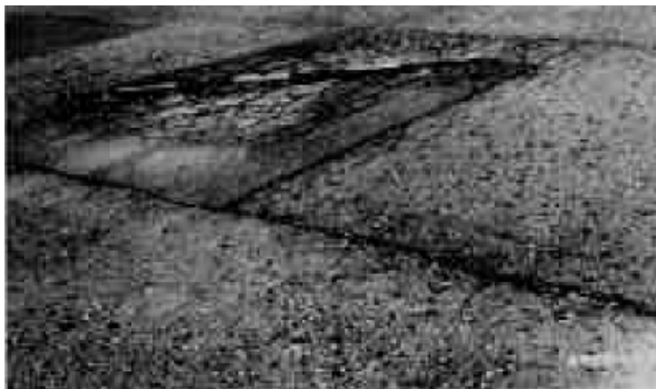
Figure A-10c. High-Severity Patching and Utility Cut Patch
