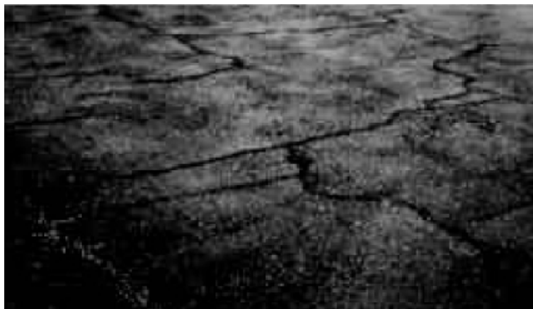
Figure A-3b. Medium-Severity Block Cracking
